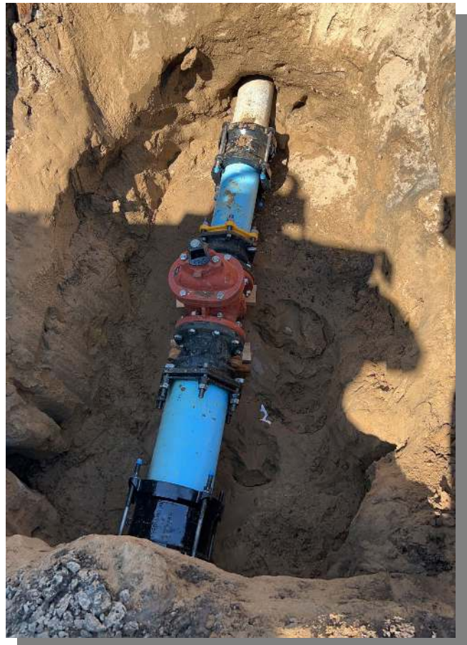
Water line valve leak on Flower Street which resulted in reducing the 8-inch valve with a 6-inch valve.
