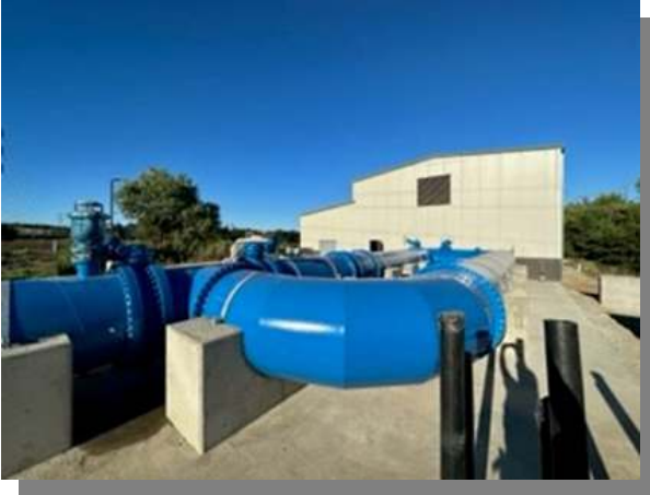
Figure 1: Raw Water Pump Station
