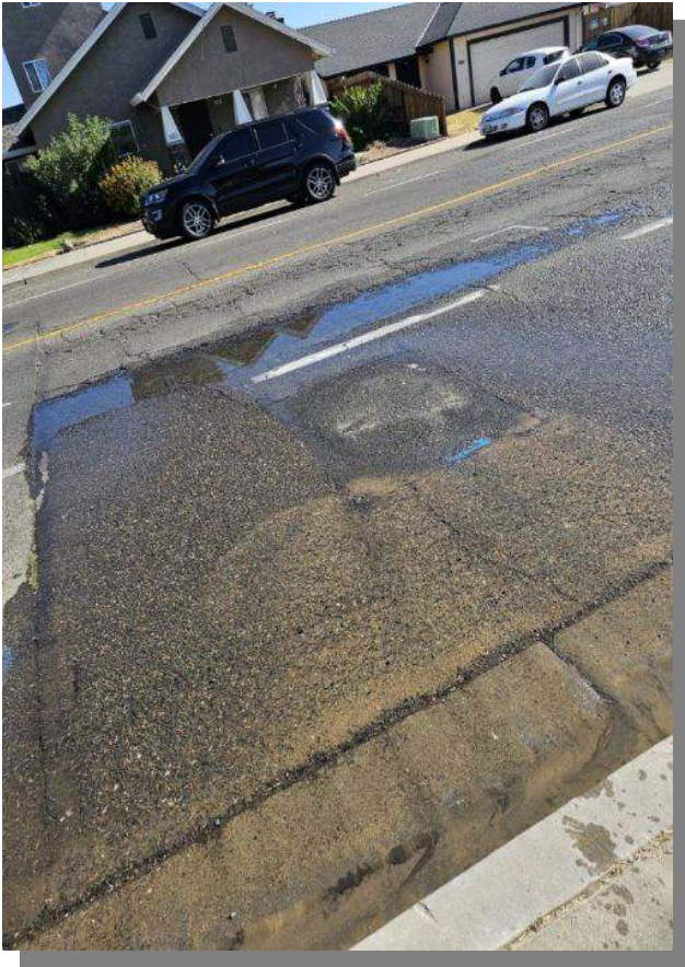
Repaired a water main leak that was causing water to come up from the asphalt on E. Linwood Ave.
